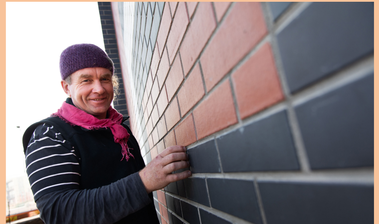
Below Artist Anton Forde at the site of the blessing and the first completed brickwork
