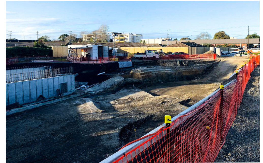
Above Digging and foundation works on the reserve's wetlands area is almost complete
